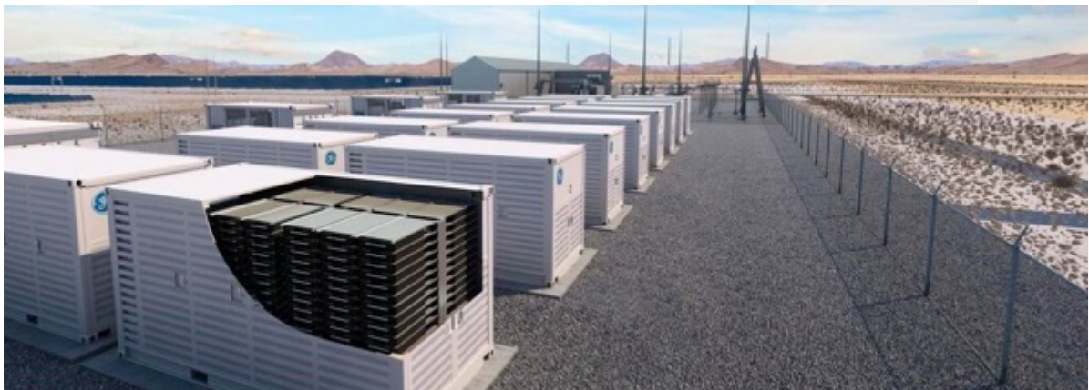
Battery energy storage systems (BESS) (eerinstitute.org)
